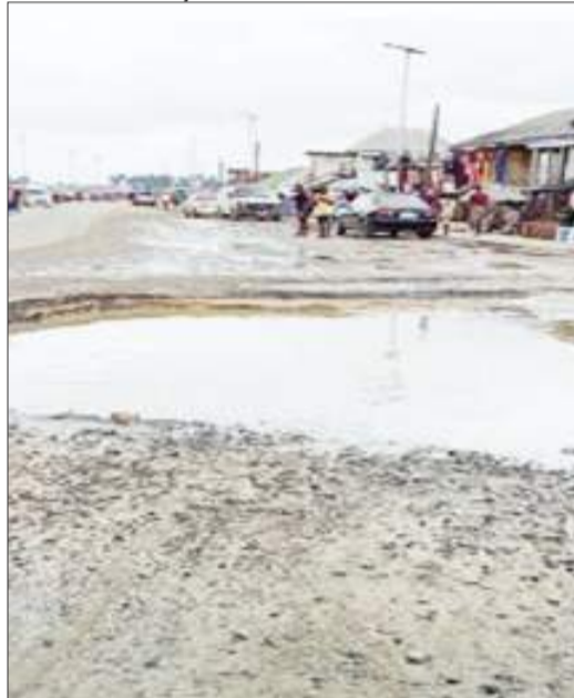
A bad road in Yenagoa
