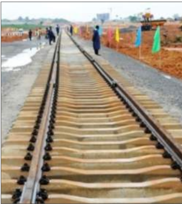
Lagos green line rail
