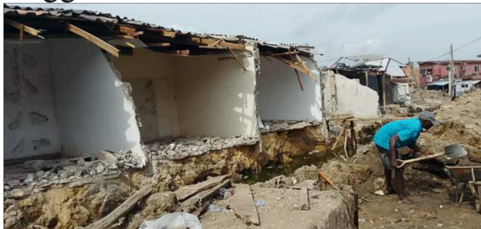
Home, shops and kiosks being demolished by the Lagos State Ministry of Works and Infrastructure
