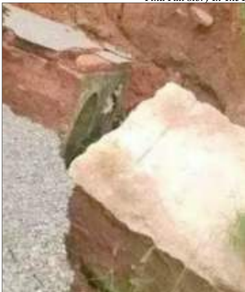
The collapsed Zagah-Suntai road
