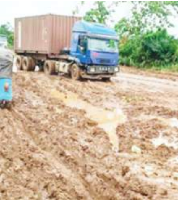
Failed Asaba-Ugbolu-illah-Ebu federal highway
