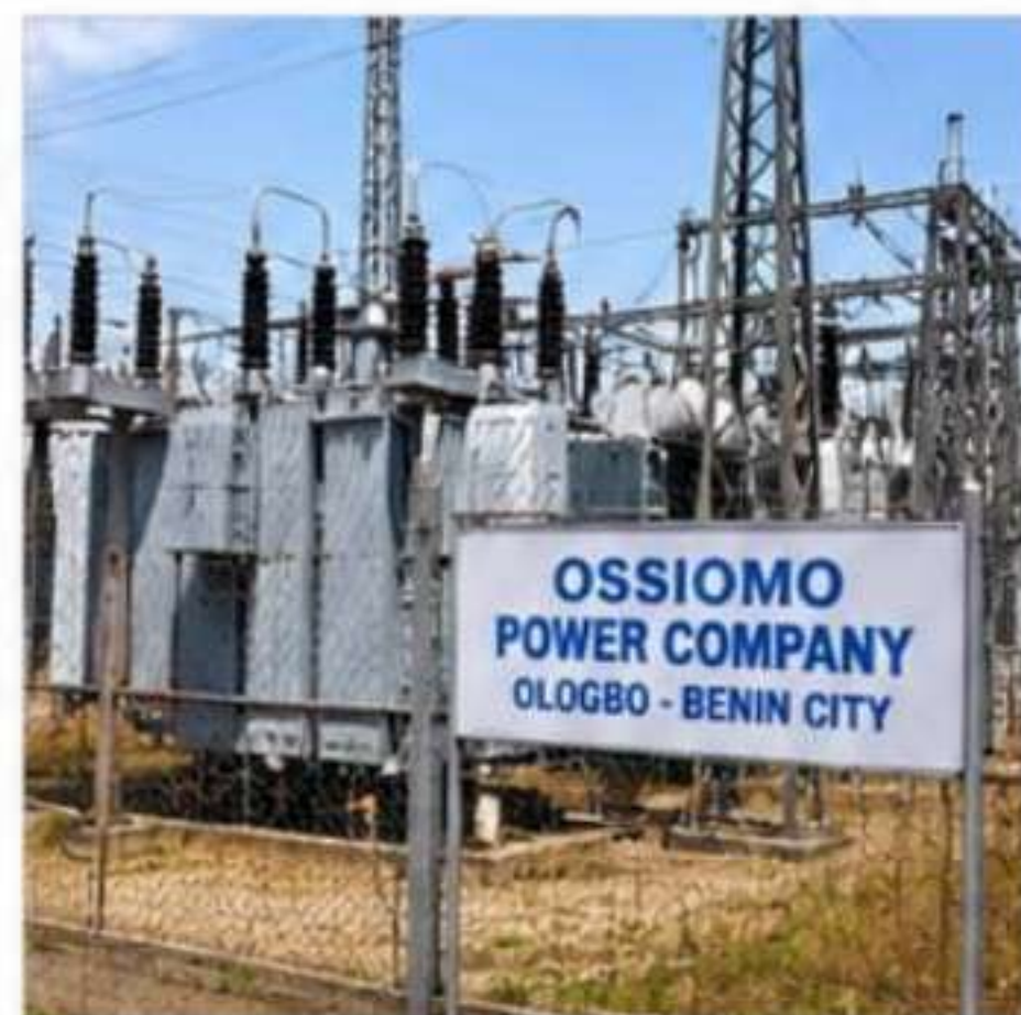
A section of Ossiommo Power Company facility in Ologbo, Benin City.
